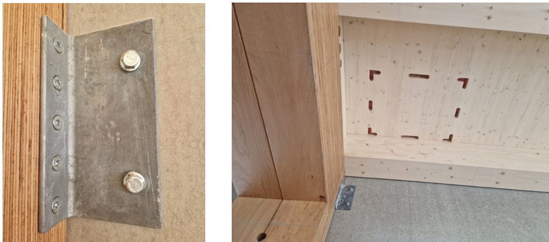
Fig. 7.2: Timber column to concrete connection with steel brackets and post-installed anchors at jobsite
