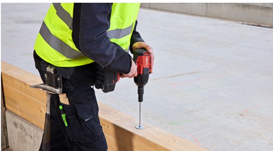
Fig. 2.3: Installation of a concrete screw anchor to fasten a timber beam to concrete directly through the timber element
