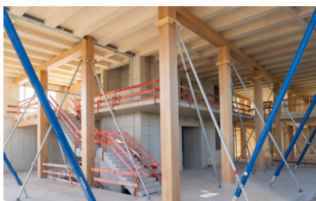
d) The primary structure (beam-column) supports timber-concrete composite ceiling system (Source: UmweltBank AG)
