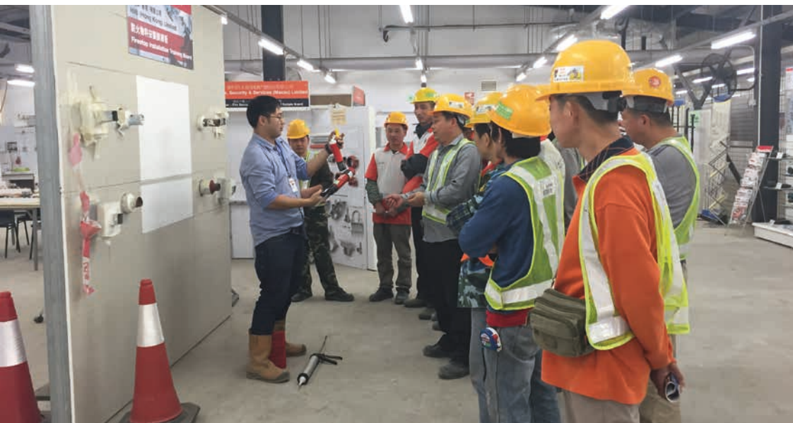
The Hilti team instructed workers on the correct way to install firestop systems directly on the construction site.
