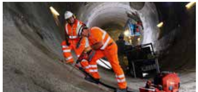
Tunnel workers are drilling their way under London. Hilti is an important partner in the project.
