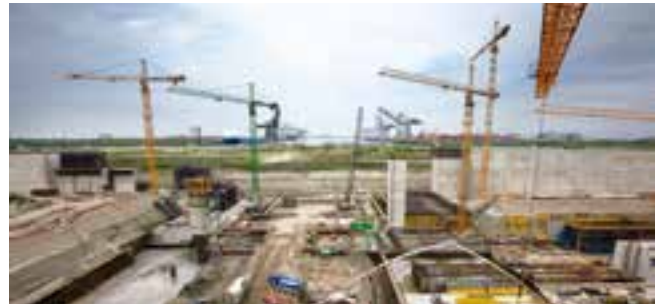
A new lock is being built in Antwerp, Belgium. Hilti is the on-site problem solver.
